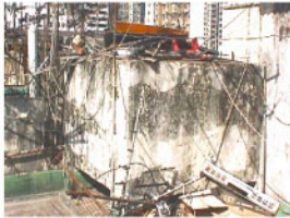
Poorly Maintained Water Tank
