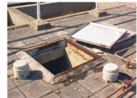
Defective Water Tank Cover
