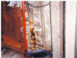
Corroded Water Pipe
