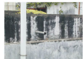
Overflow Pipe without Lid
