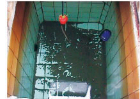
Dirty Water Tank
