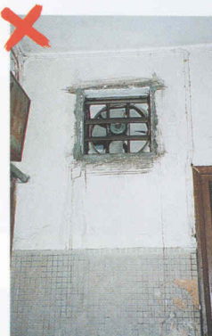
Unauthorized opening in fire resisting wall and the installation of exhaust fan
