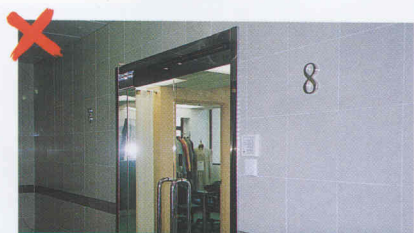
Door of inadequate fire resistance opens onto common corridor
