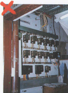
Unprotected electric meter room
