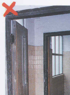
Damaged / Missing fire doors
