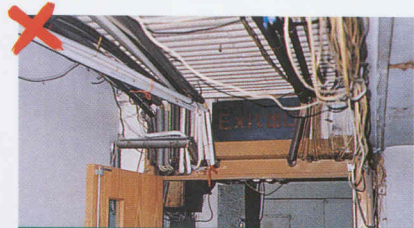
Services within staircase enclosure without proper protection
